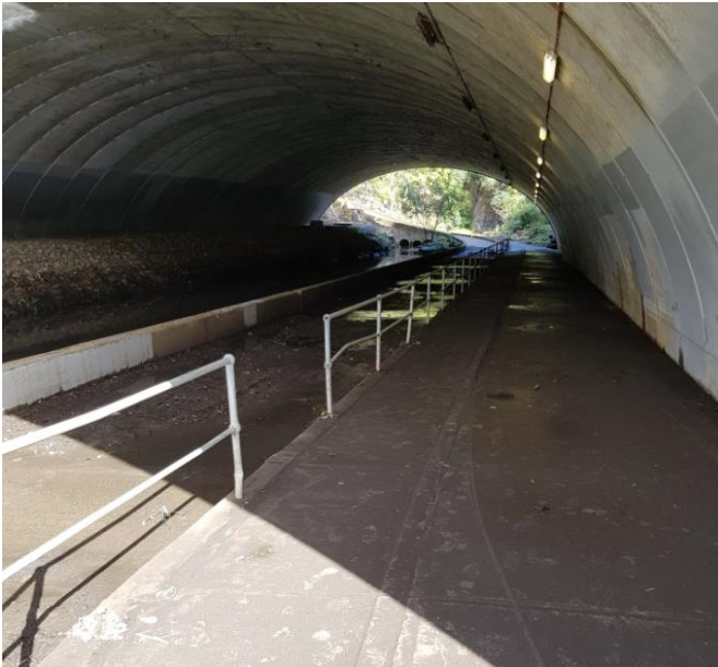
Figure 72 - C3-3 Sewage Overflow and Stormwater- Sutherland road underpass looking south west
