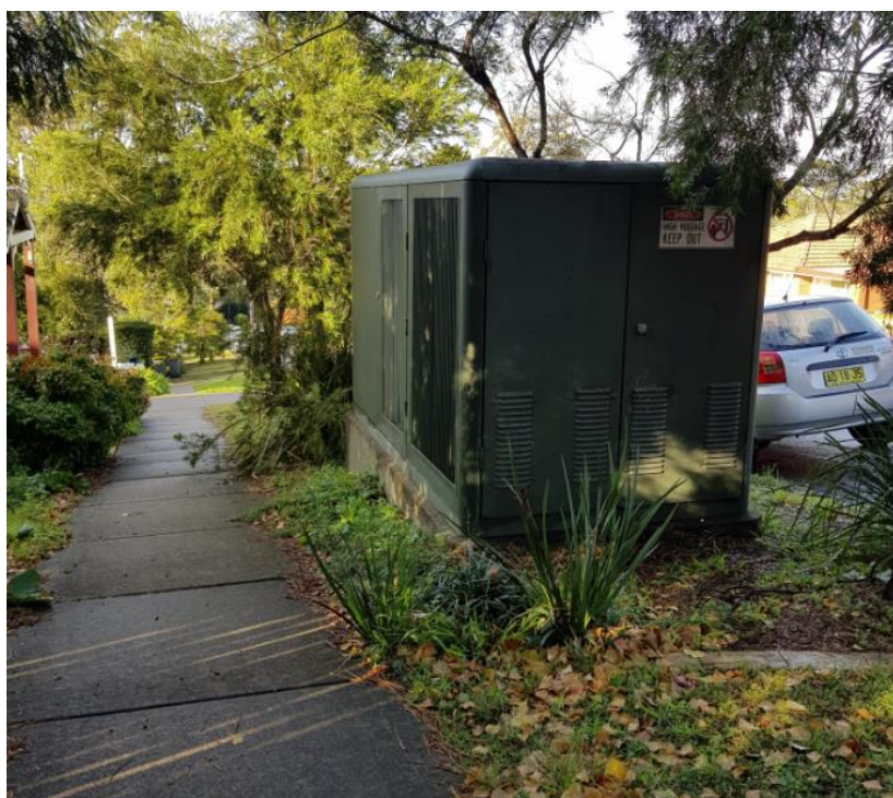
Figure 13 - A1-9 High Voltage Power Box - Looking south east along Lilla Road
